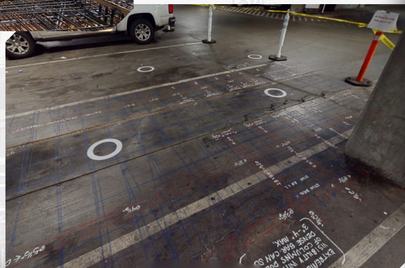
3D camera image capturing as-built conditions and concrete scan markings for a parking garage renovation.
