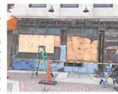
The exterior of Bell Pharmacy was once covered in stucco, but its large windows and original signage will soon be restored. COURTESY OF TONY MINNITI
