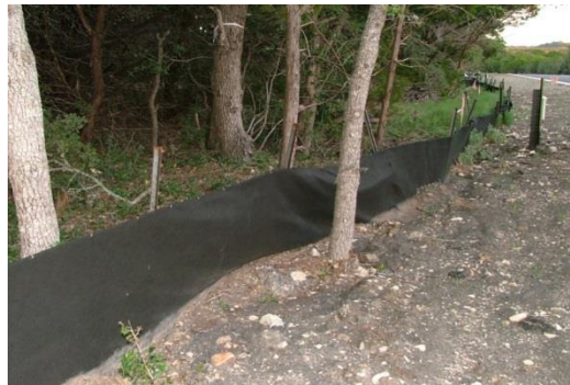
Temporary Silt Fence
