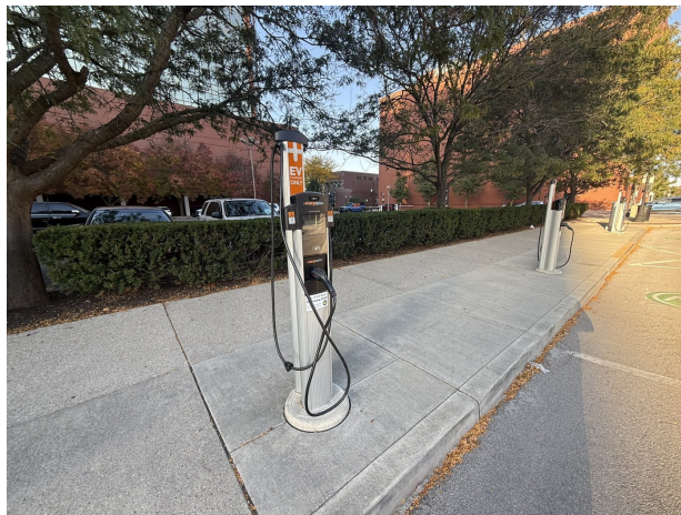
Driving electric? ChargePoint EV charging stations are right along Berry Street, steps from the building.
